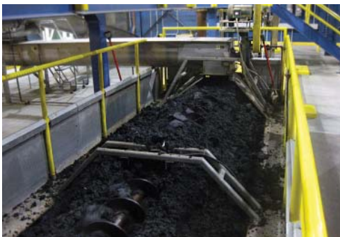
Biosolids moving from the centrifuge to a truck for transport.
